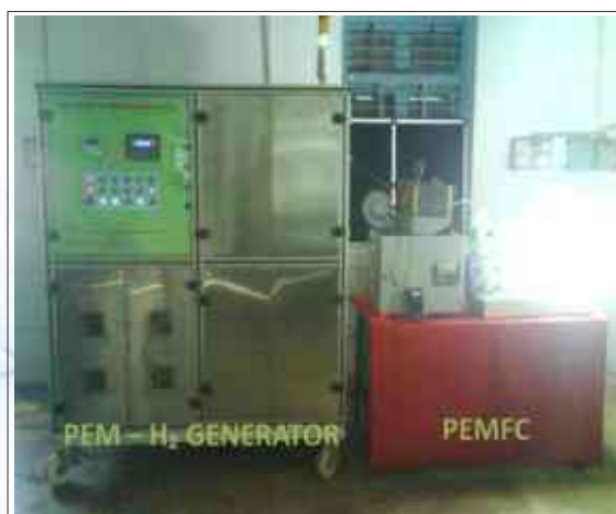
Integration of 1.0 Nm 3 /hr PEM Water Electrolyser and PEM Fuel cell
