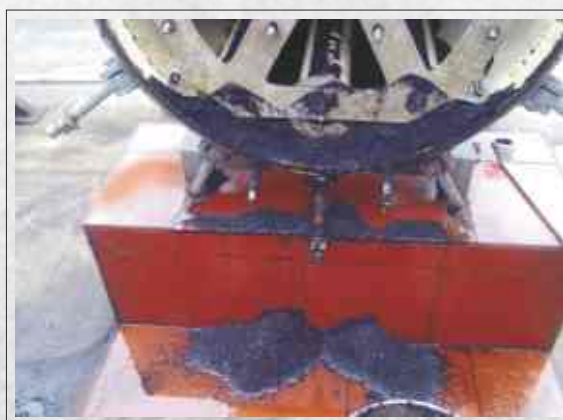
Corrosion product in the pipeline
