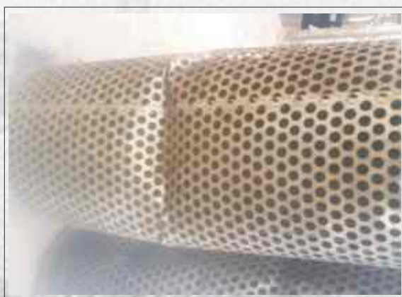
Filter damage in ATF pipeline
