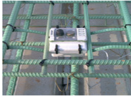
Figure 10. ECI sensor during operation
