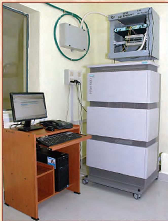
Newly Installed Central telephone facility Siemens HiPath 4000 V5.0
