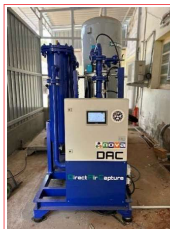
Figure 1. Direct air capture unit installed at CECRI.
